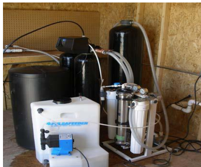
Reverse osmosis system installed in the eastern Coachella Valley
