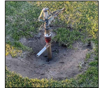
Manual Sprinkler from 1960's
