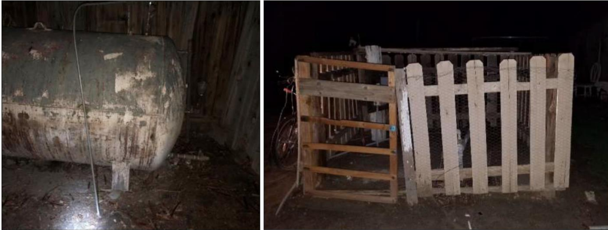
Figure 3-16: Pressure Tank (left) and Well with Fencing (right)
